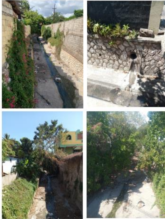
Figure 4-43 Gully Network and Adjacent Vegetation in the Project Vicinity
