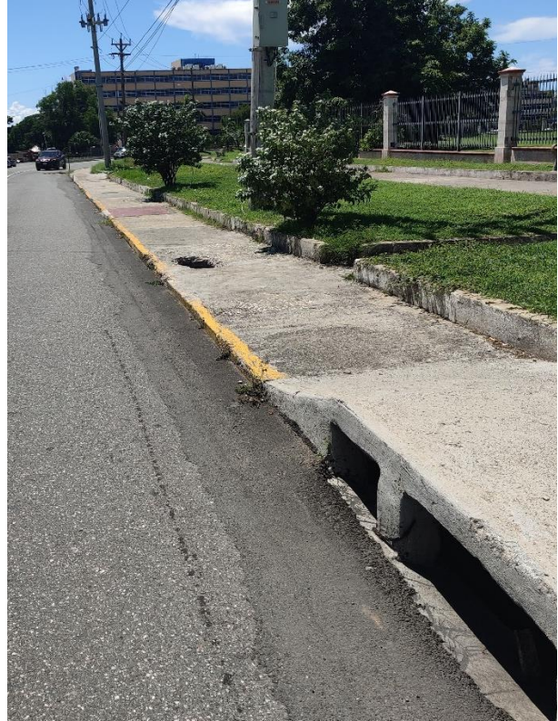
Figure 4-13: Inlet leading to underground drainage system
