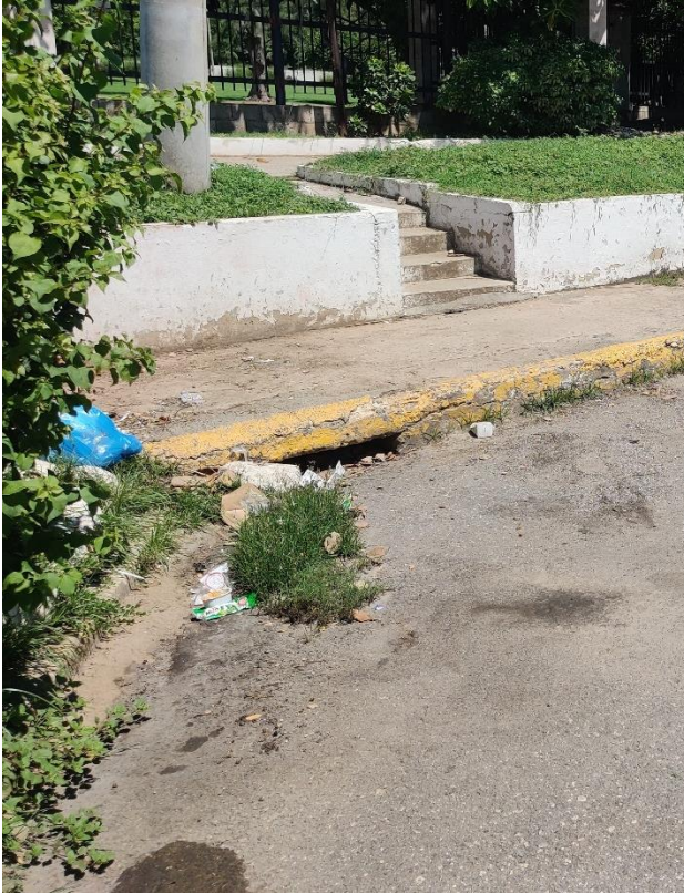
Figure 4-14: Inlet leading to underground drainage system
